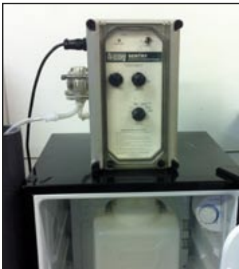
Installed on a standard undercounter refrigerator drilled for inlet hose
